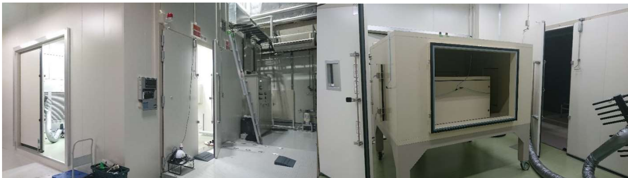
Next generation dynamic performance evaluation facility
